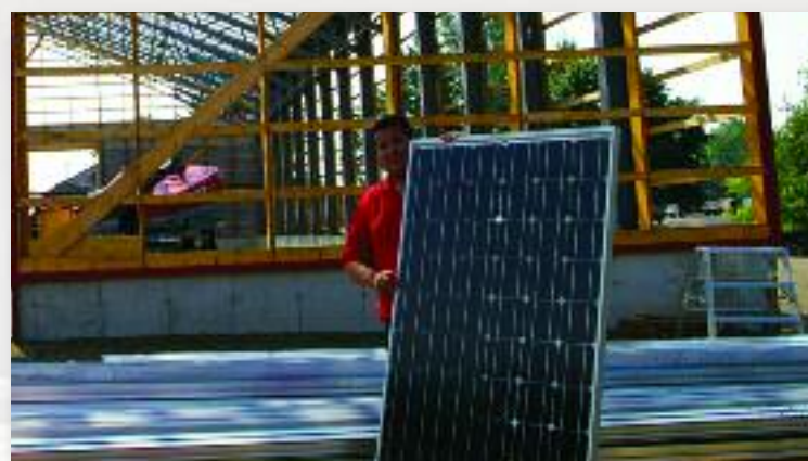
Home Owner Michael McDonald shows off the Galaxy Solar Panel.
